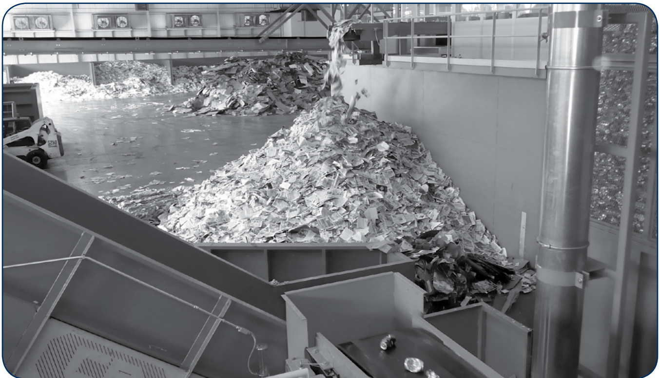
Pictured above is the interior of Horry County's material recovery facility – an example of a publicly owned MRF.
