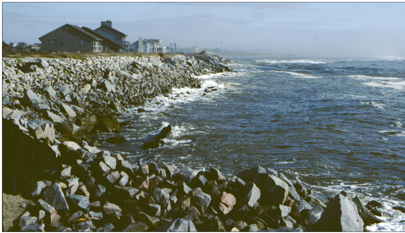
FIGURE 33.6. Beach erosion along North Beach led to exposed seawalls, no recreational beach, and severe damage to structures in 1983. View north along Renken Point in 1985 at low tide. [After CSE 1989]
