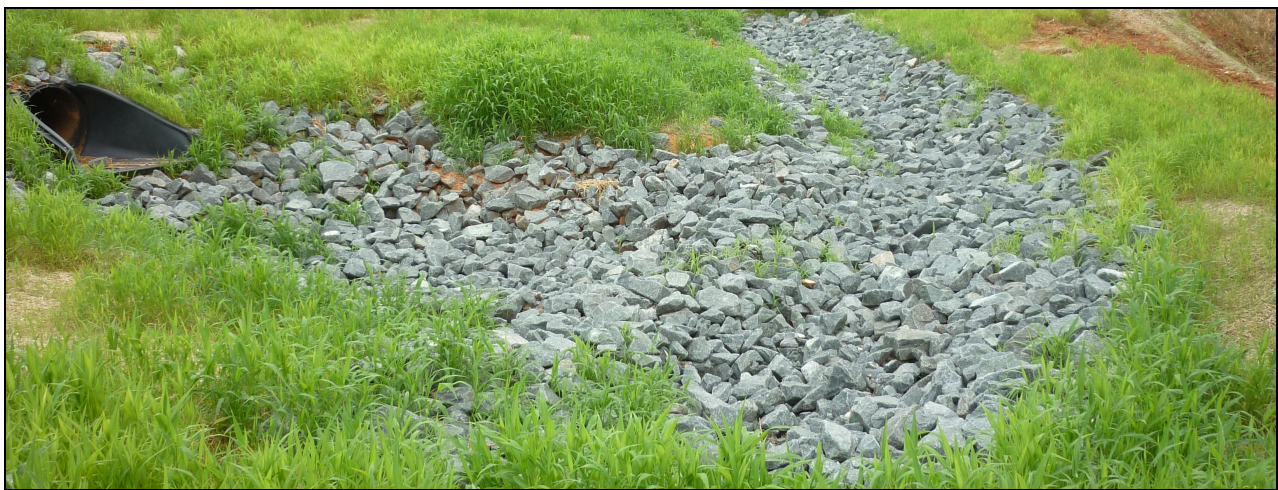
Photo: Principle Spillway's Barrel (Outlet Pipe) with Plunge Pool and Level Spreader
