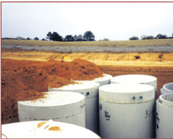
Cylindrical B/C Trench disposal vaults in an active trench. Vaults are immediately backfilled to fill void spaces and reduce radiation exposure.
