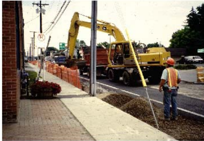
NY State Dept of Transportation installation of CU Structural Soil in Ithaca,, NY 1997. Fifty trees of five species planted into continuous trenches.
